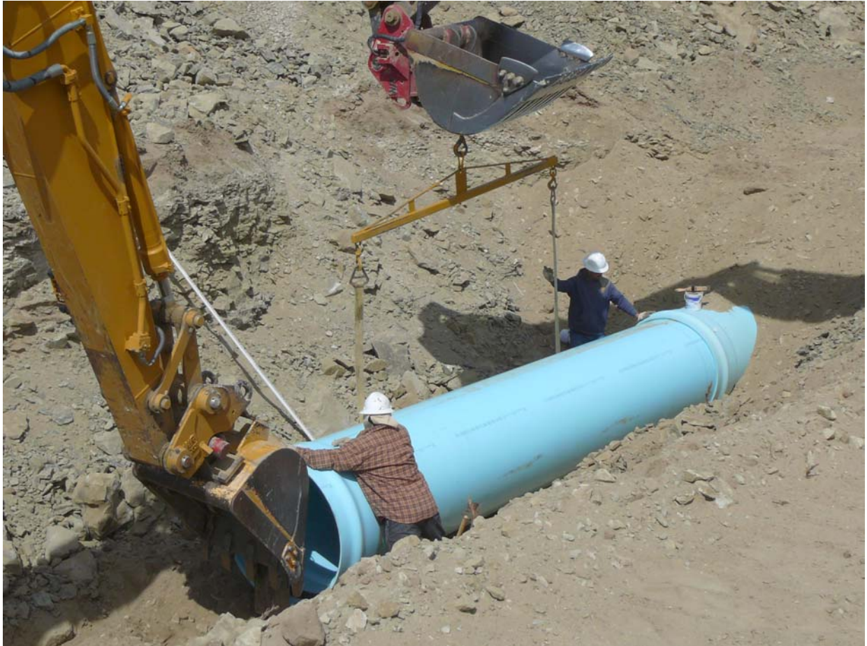
Figure 8. District Construction Crew Installs 42 inch PVC Mainline on Hidden Valley Pipeline Project
