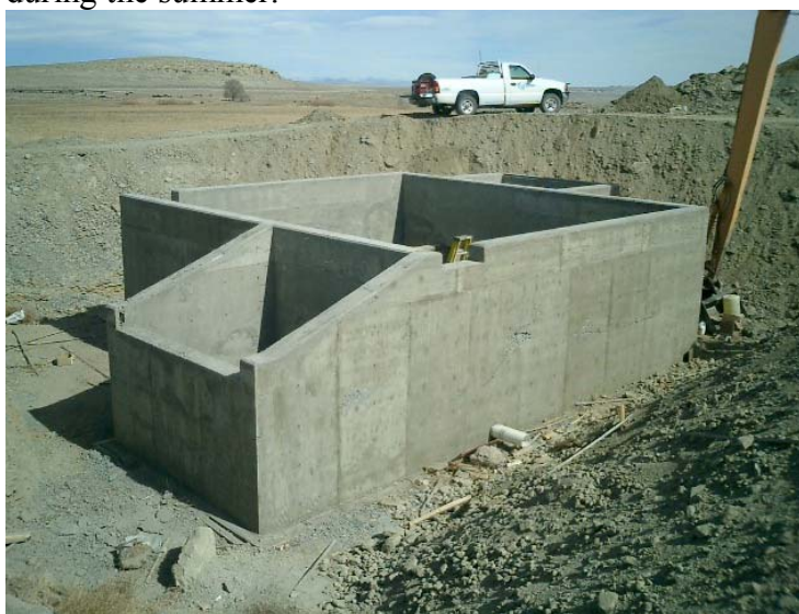
Hidden Valley Pipeline Inlet Structure
